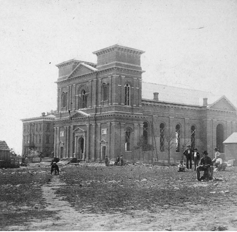
1.2 Cathedral of the Immaculate Conception at Leavenworth during construction in 1867. Courtesy of KansasMemory.org, Kansas State Historical Society, Copy and Reuse Restrictions Apply
